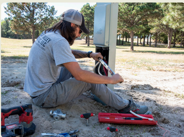
Robert Osbon of North Platte connects new electric lines to a pedestal to upgrade service in the Cedar Bay Campground at Merritt Reservoir State Recreation Area in Cherry County. ERIC FOWLER, NEBRASKALAND
