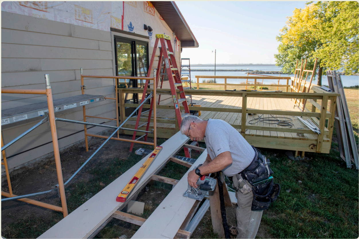
Mark Crosby of the Nebraska Game and Parks Commission cuts siding for the Pawnee Marina concession and University of Nebraska-Lincoln Rowing Club building, a partnership project. The renovation was paid for with the Capital Maintenance Fund. The renovated building will be home to Game and Parks offices, a classroom for hunter and boater education, and be the UNL Rowing Club practice facility. ERIC FOWLER, NEBRASKALAND
