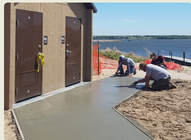
A new bathroom and sidewalk compliant with the Americans with Disabilities Act are finished at Buckshot Bay boat ramp at Calamus Reservoir State Recreation Area. JOHN IRONS, NEBRASKA GAME AND PARKS COMMISSION
