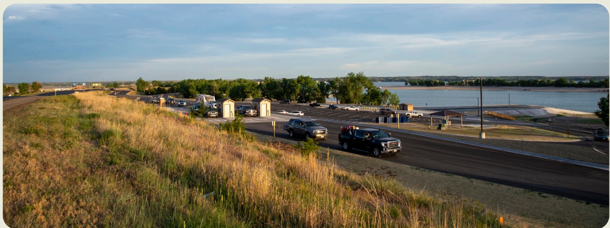
A new entrance to Martin Bay at Lake McConaughy State Recreation Area in Keith County was completed in May of 2022. The project will improve access and traffic flow at the park's most popular entrance. The project was partially funded by the Nebraska Game and Parks Commission's Capital Maintenance Fund. ERIC FOWLER, NEBRASKALAND
