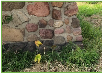
Stone Shelter House high water stain, 2020
