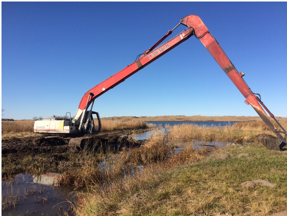
Picture from Juancarlos Giese of excavation at the VNWR Aquatic Habitat Project
